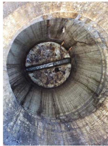
MH1228 – Infiltration Stains
