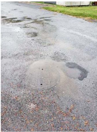
MH 2042 – Stormwater Entering Vent Hole
