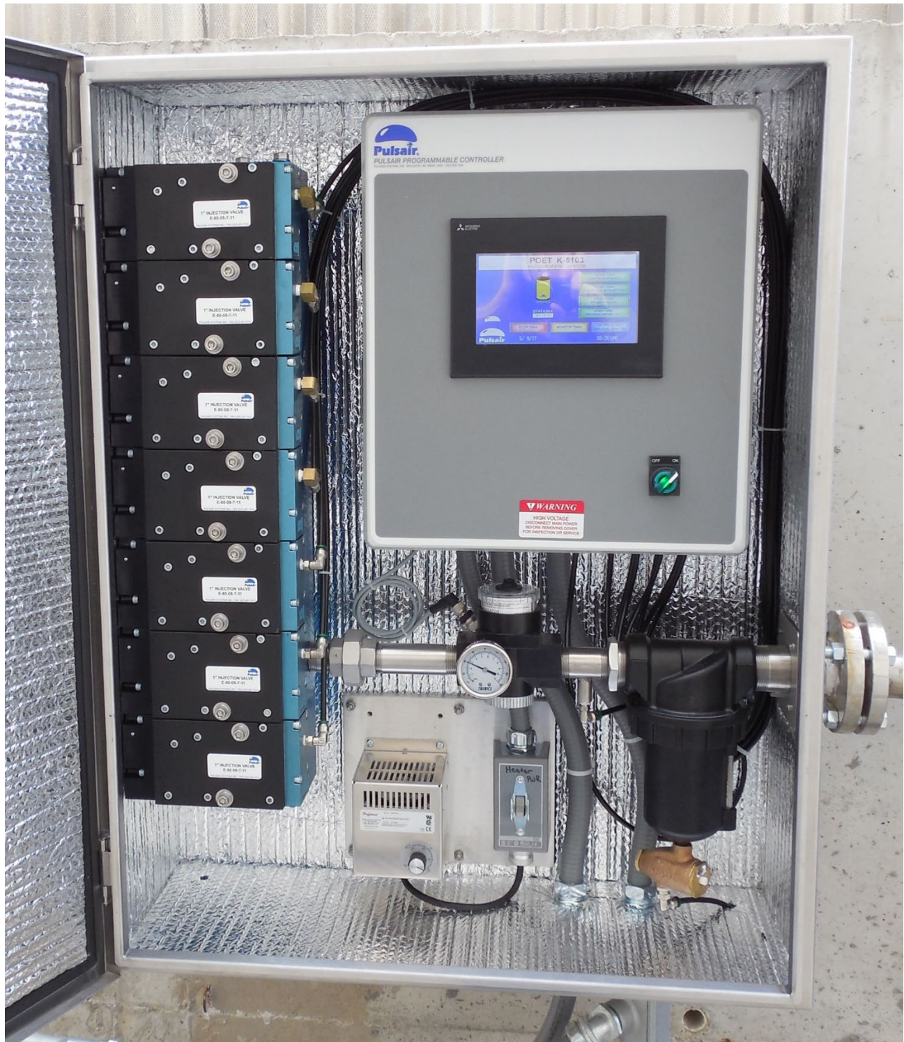
Example image of PPC Mixing Controller inside valve enclosure
