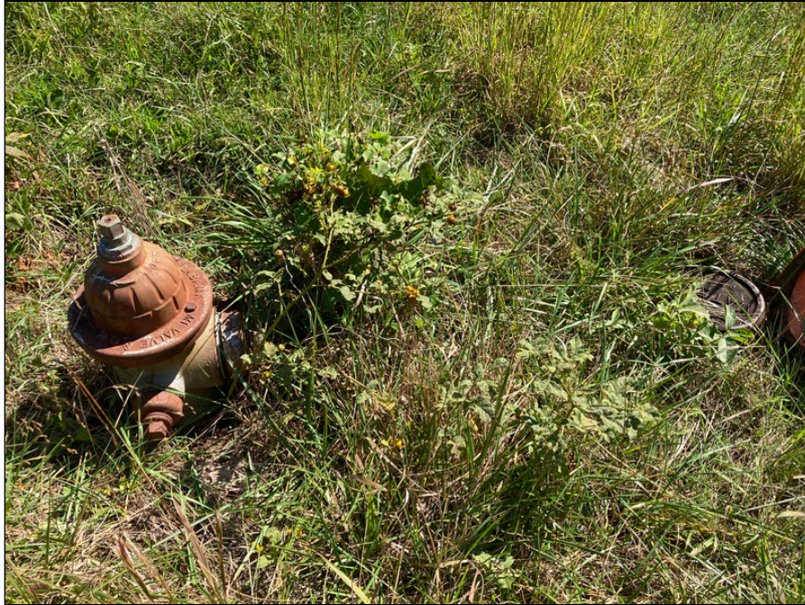
13 - Fire hydrant and water main access point
