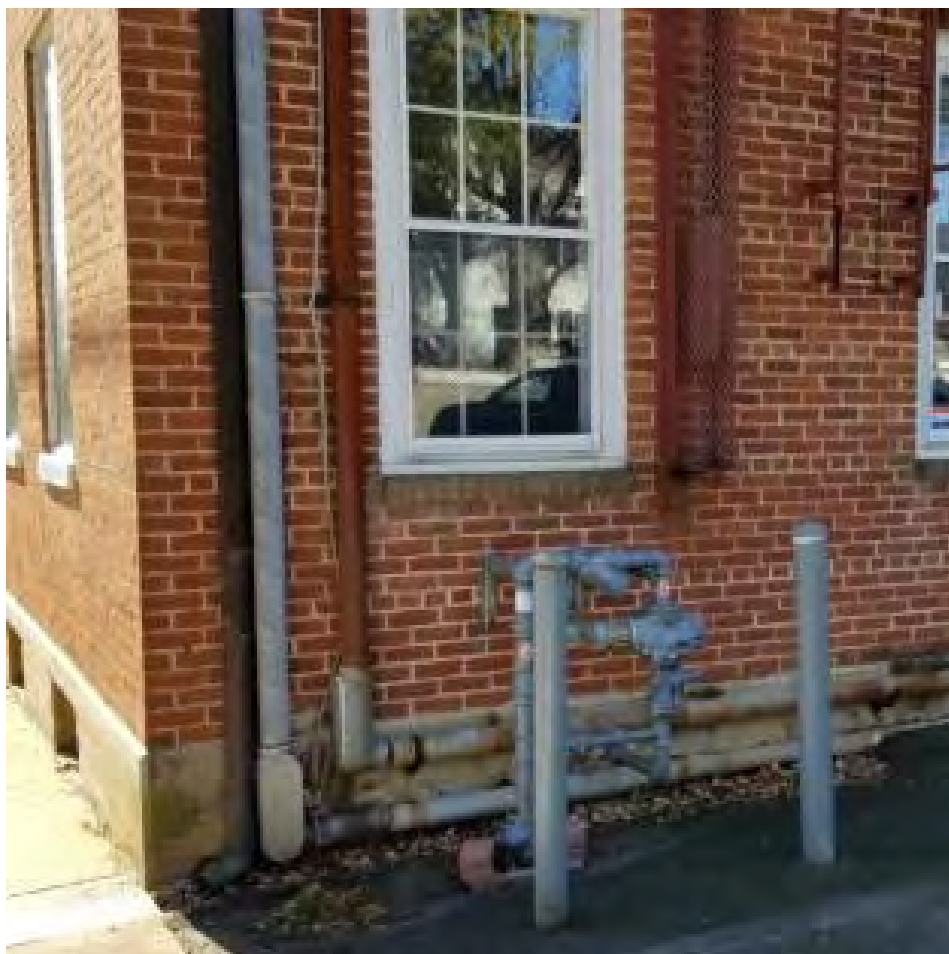
Figure 3-70: These utility lines and meters are appropriately located at the back of the building. The conduit lines are painted to match the building.
