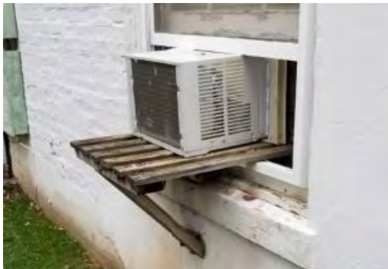
Figure 3-65: This window air conditioning unit is located at the rear of the building and is not permanently attached to the structure. Though unsightly, it meets the intent of the historic district guidelines.
