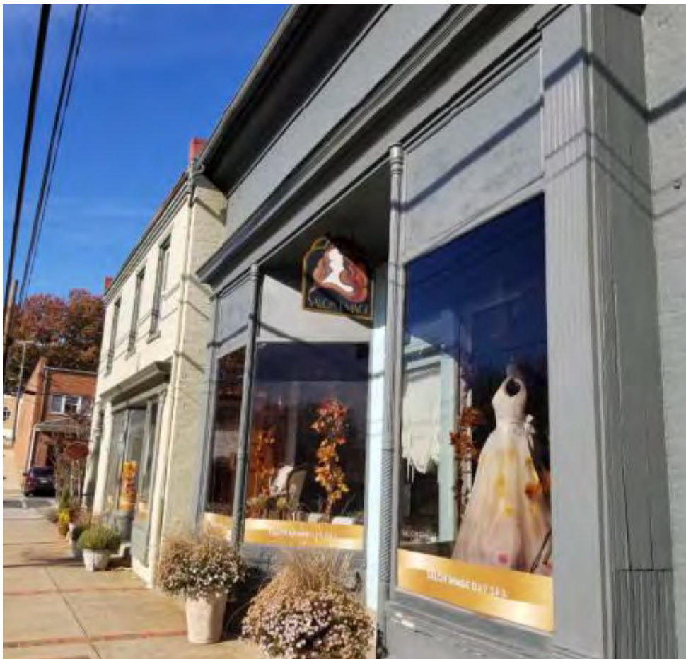
Figure 3-34: This storefront retains its original form, including cornice and entablature, its recessed entry, and its wood framing. The transom panels, however, have been clad with plywood, which is not appropriate.
