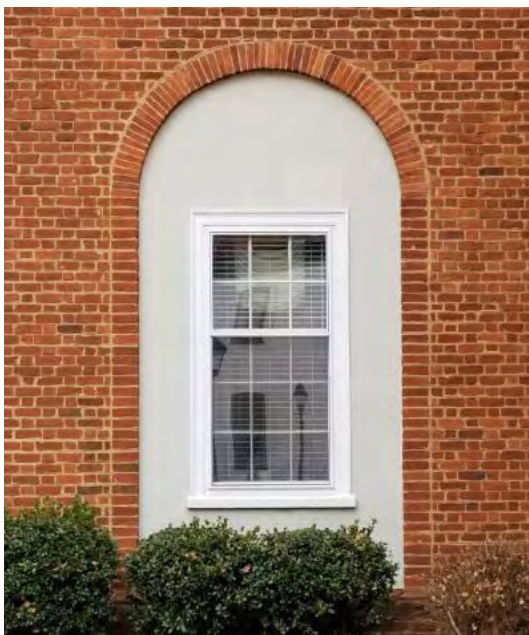
Figure 3-29: Windows should properly fit their respective fenestration openings as they do at the Main Street post office (above). The window below looks awkward; the fenestration opening should be fitted with more appropriate glazing.
