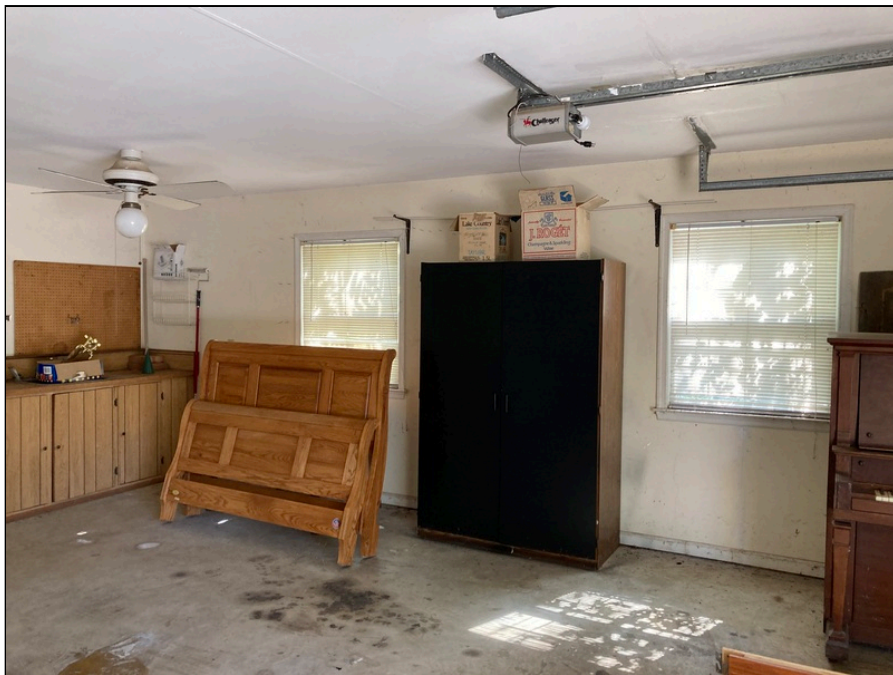
34 - Garage with de minimis staining
