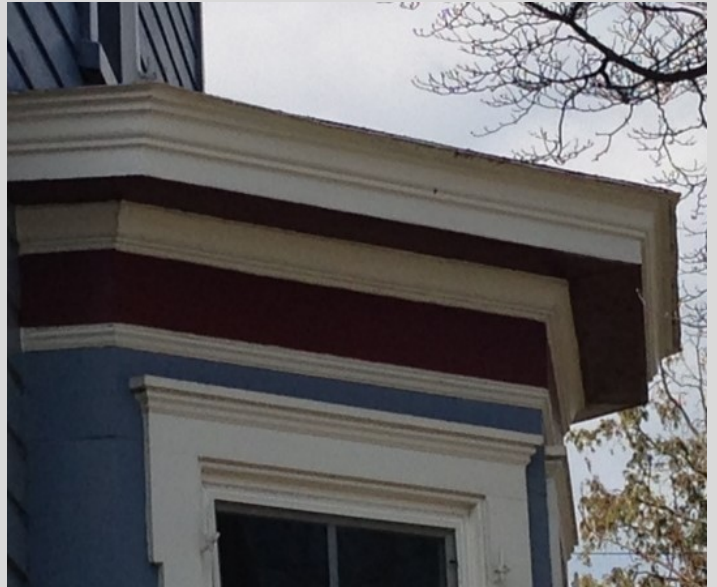
Illustration 5: Above is a good example of well maintained cornice to a residential house in the Historic District.
