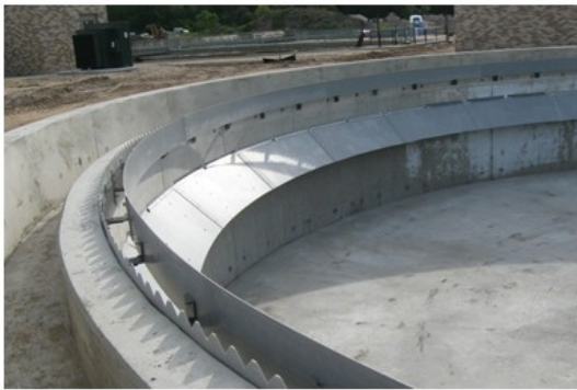
Weirs, Scum Baffles & Density Current Baffles
