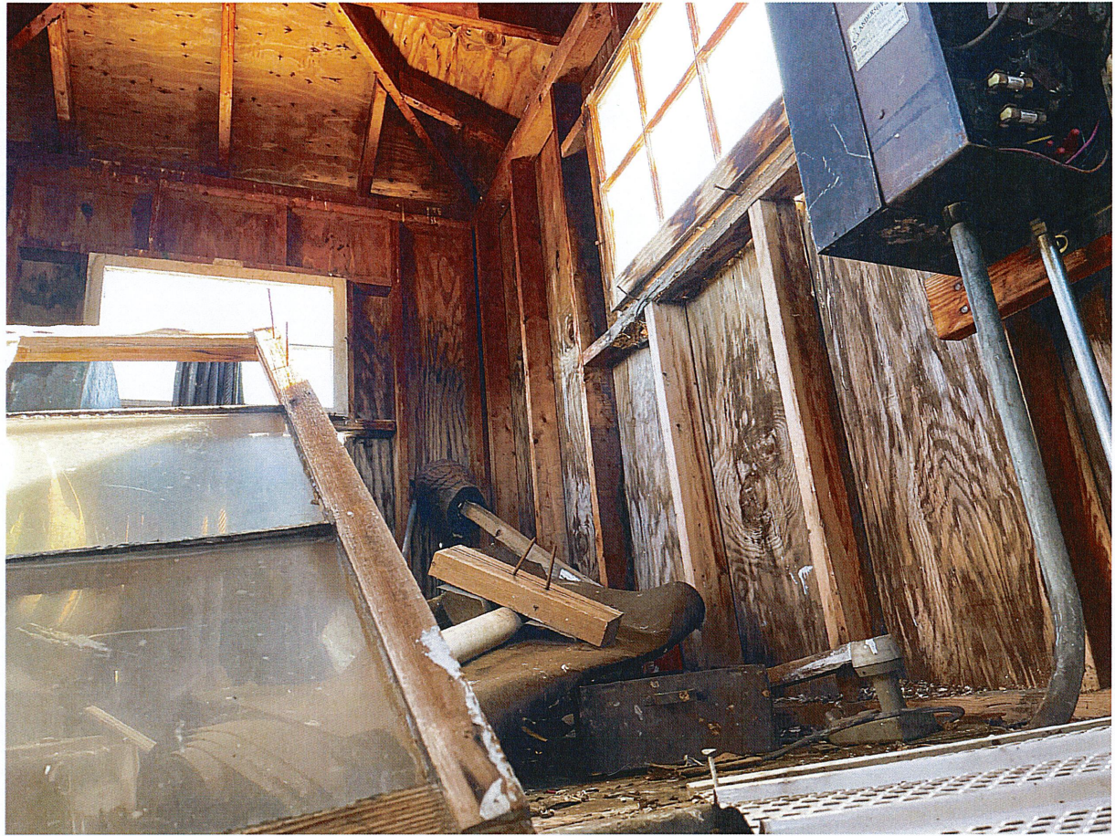
Photo 3 – Damaged Penthouse Floor Structure
