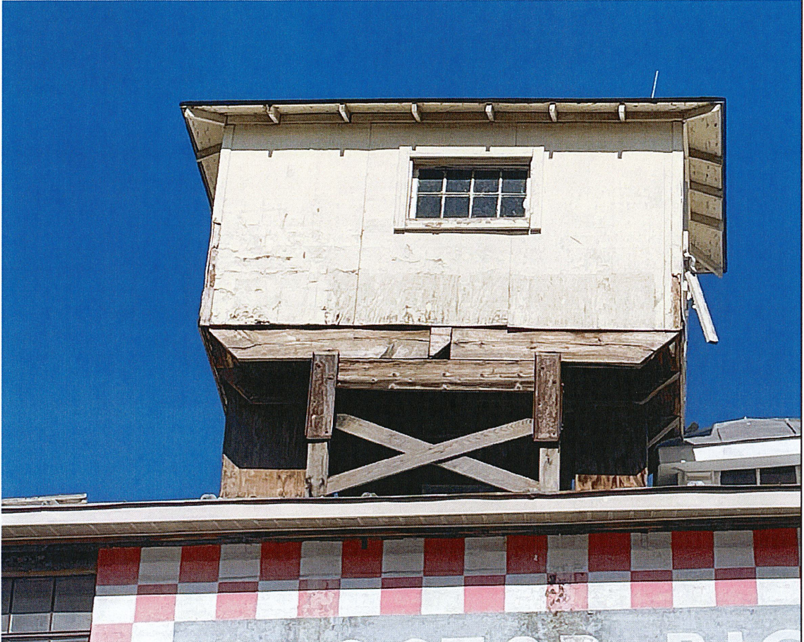
Photo 2 – Ineffective steel channel braces
